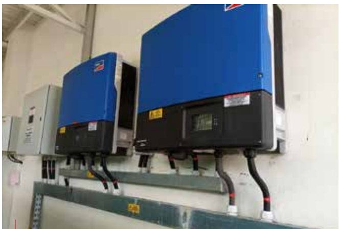
Inverter installations at TOTAL service stations
