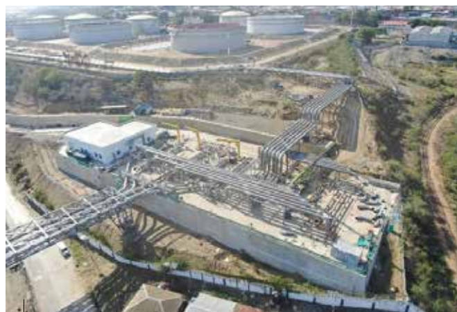
Beach Valve Station area (S4)
