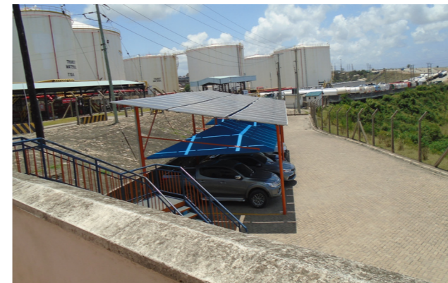
Solar PV panels installed to provide renewable power to the office building.
